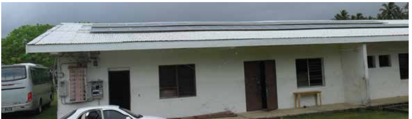
The 10kW array on the Lycee de Luganville in Sanma Province, Espiritu Santo, Vanuatu
