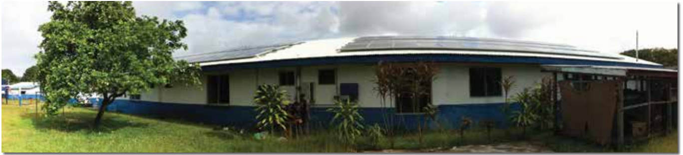
The 20kW array on the Hospital in Sanma Province, Espiritu Santo, Vanuatu
